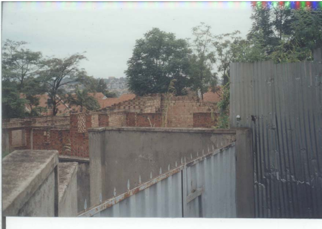
The incomplete structure at plot 102 Luthuli Avenue ( excluding the Gate and the concrete wall)
